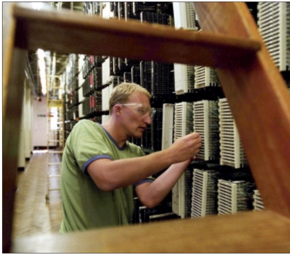
Unbundling a local telephone exchange and making ready for ADSL. (Picture courtesy of BT and VisualMedia)
